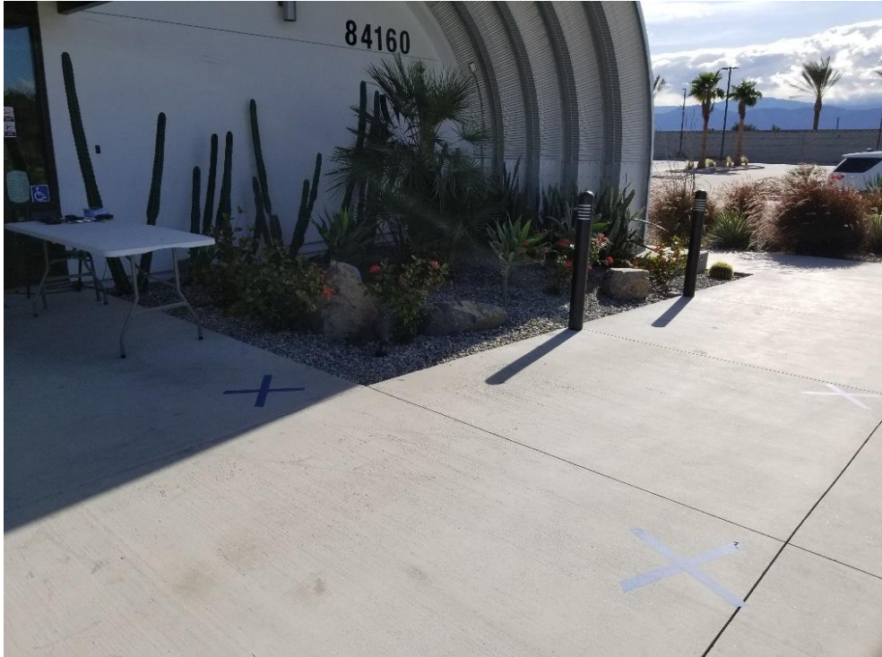
“Blank Wall Façade” is missing required additional glazing
